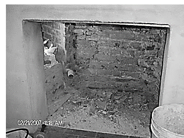
Badly Deteriorated Firebox
