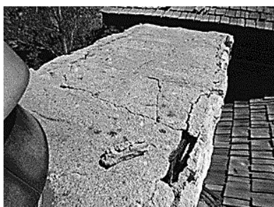
Damaged Chimney Cap
