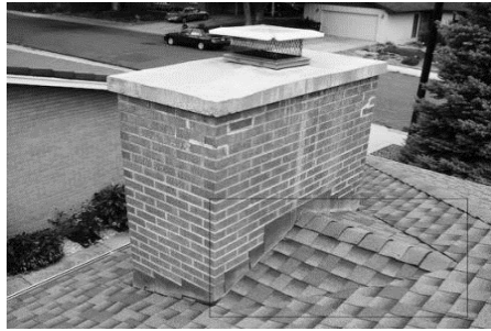
Clay Liner Cover
